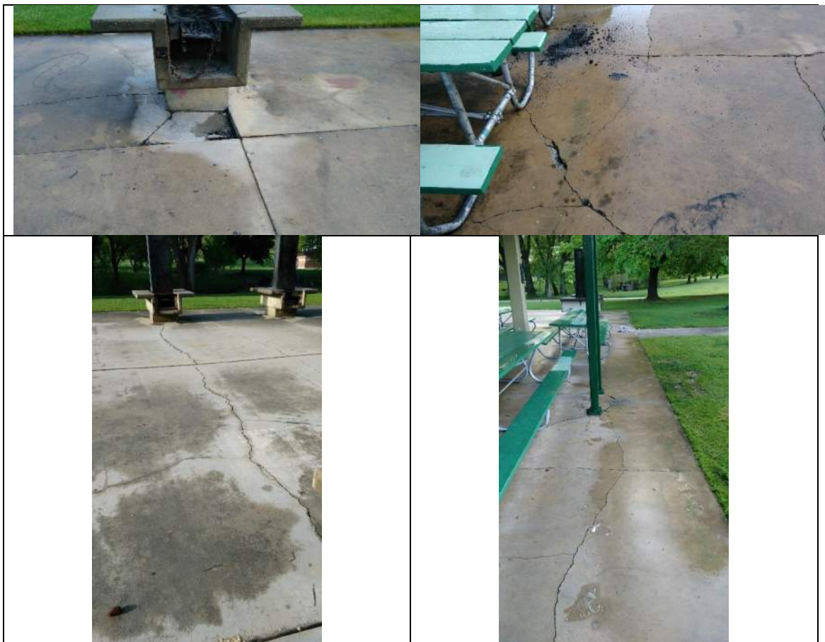
Figure: Representative Cracking Examples
